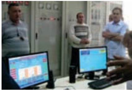
Tajik delegation gets acquainted with the operation of the small hydropower station at Aghstev river, June 2011 (Bilorom Saidova)
