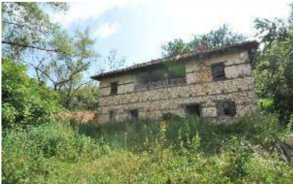
Figure 16 – Abandoned vernacular homes could be adapted into guest houses. Photo: Rand Eppich
