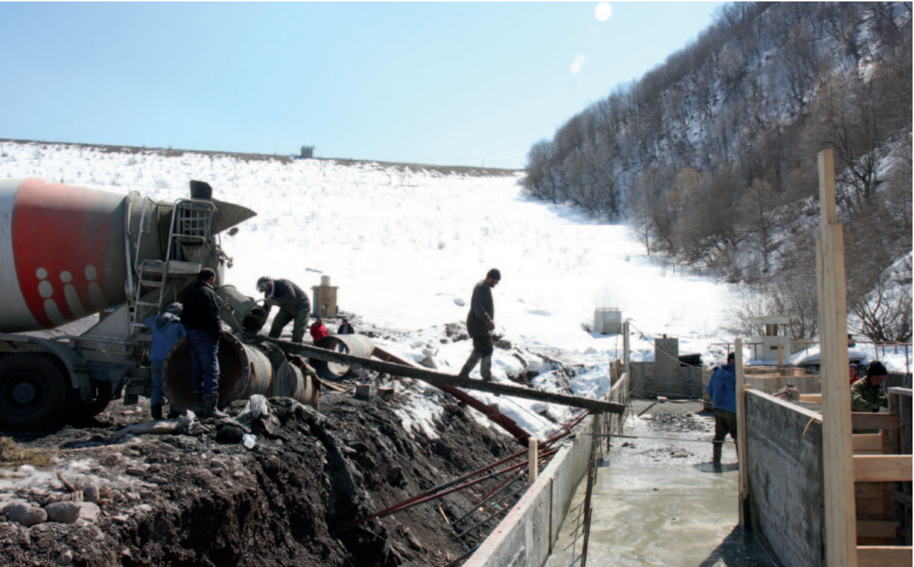
Refurbishment of the right wing of the service outlet of the Zonkari Dam. March 2012. (OSCE/ Emmanuel Anquetil).
