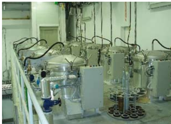
Figure 6.1: Melt out of TNT with autoclaves at munition disposal factory Ankara (courtesy NAMSA)
