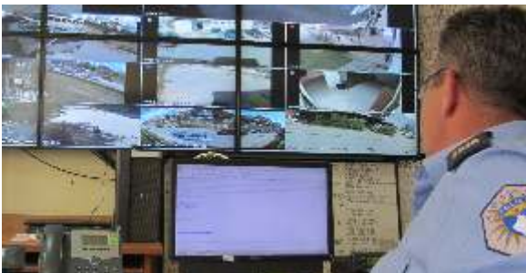
Control room in Ferizaj/Uroševac RDP
